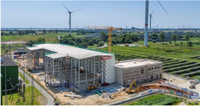
Figure 3: BorWin6 converter station in Büttel. Credit: TenneT [3]
